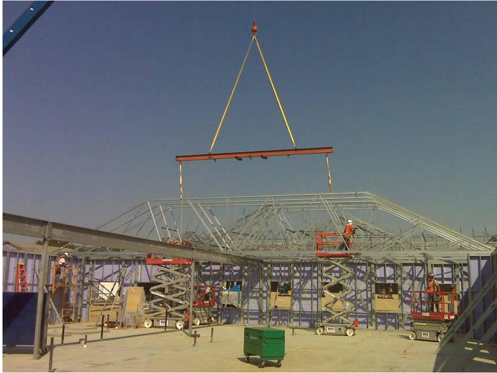
Alpine TrusSteel trusses can be set one truss at a time as shown above
