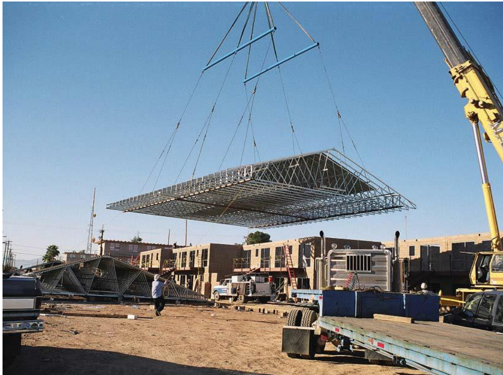
TrusSteel trusses can be assembled on the ground with the whole roof set in place at one time
