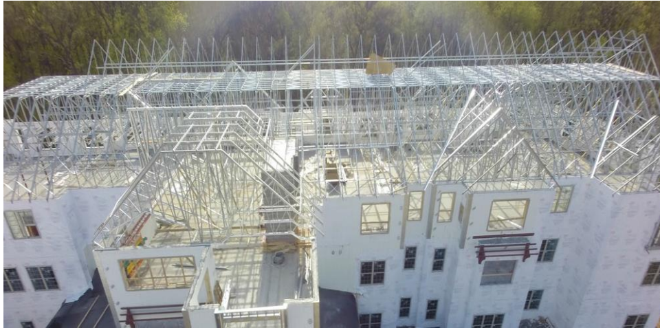
Roof framing with metal trusses from Alpine TrusSteel, a three-story, 67-unit assisted living center
