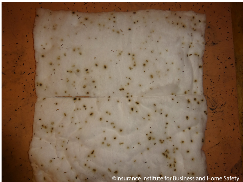
Figure 19. A cotton pad positioned on the attic floor at the base of a gable end vent showing numerous ember strikes. The cotton exhibited short-term smoldering combustion, but always self-extinguished without transitioning to flaming combustion.
