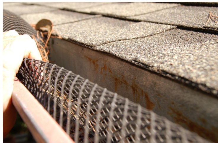
Figure 6.5 Metal drip edge installed at the edge of the roof. In this case, the drip edge was part of the gutter. Photo: Stephen L. Quarles
