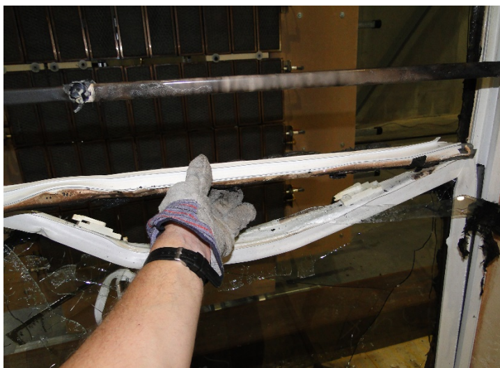
Figure 7.1. This window frame was exposed to radiant heat. The metal-reinforced member (in the back) did not deform when exposed during the exposure interval. The member without the metal reinforcement deflected downward, allowing insulated glass unit to fall out (without initial glass breakage), exposing the interior of the home. Photo: IBHS.
